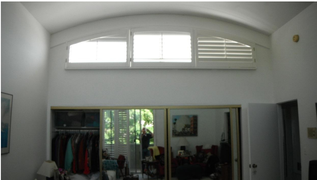
The window area that may be leaking, check with the h.o.a.
