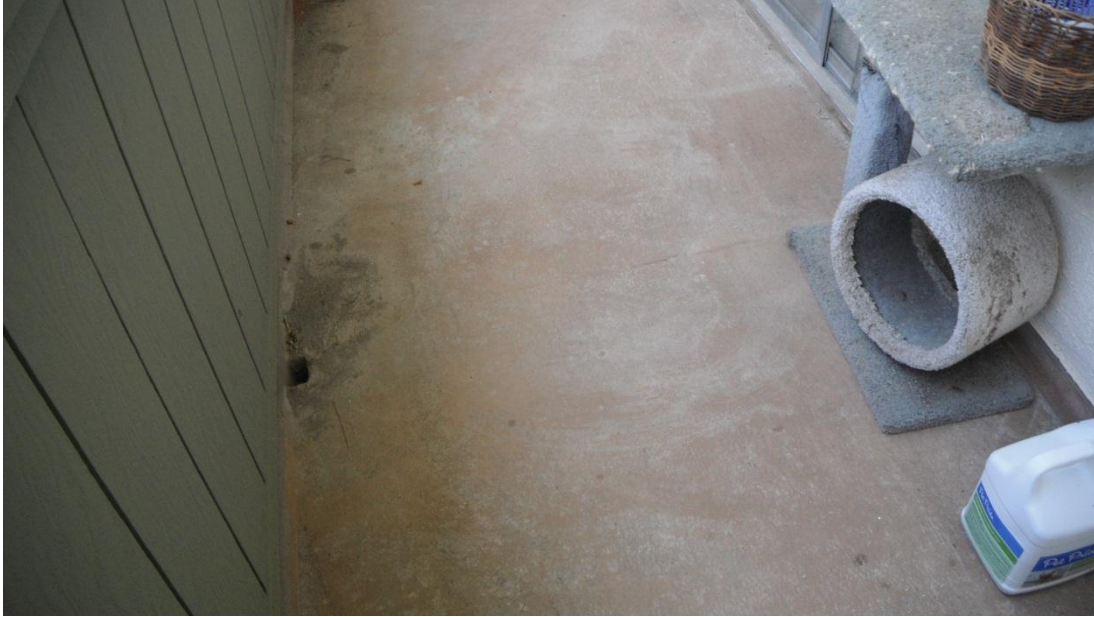
Cracks in the upstairs master bedroom exterior deck area.
