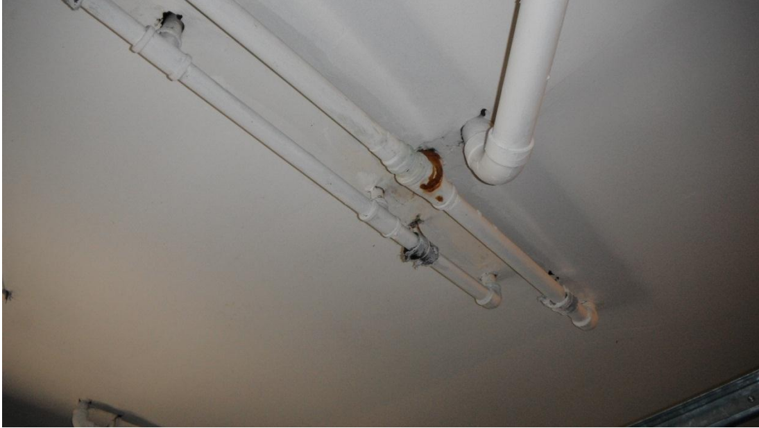
Leakage in the garage area galvanized pipes.
