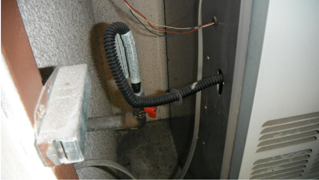
The furnace and flexible connector that is not protected.
