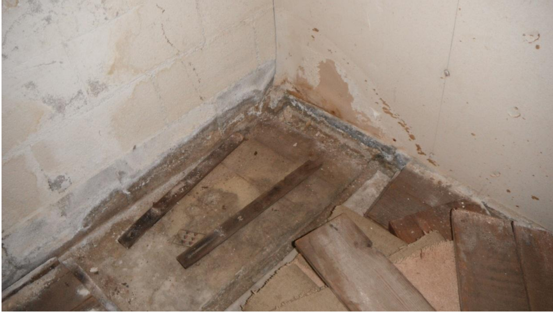
Underground water seepage. Check with the h.o.a.
