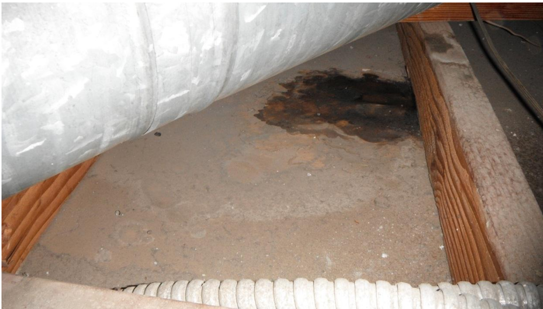
A leaking water pipe in the attic above the entry.
