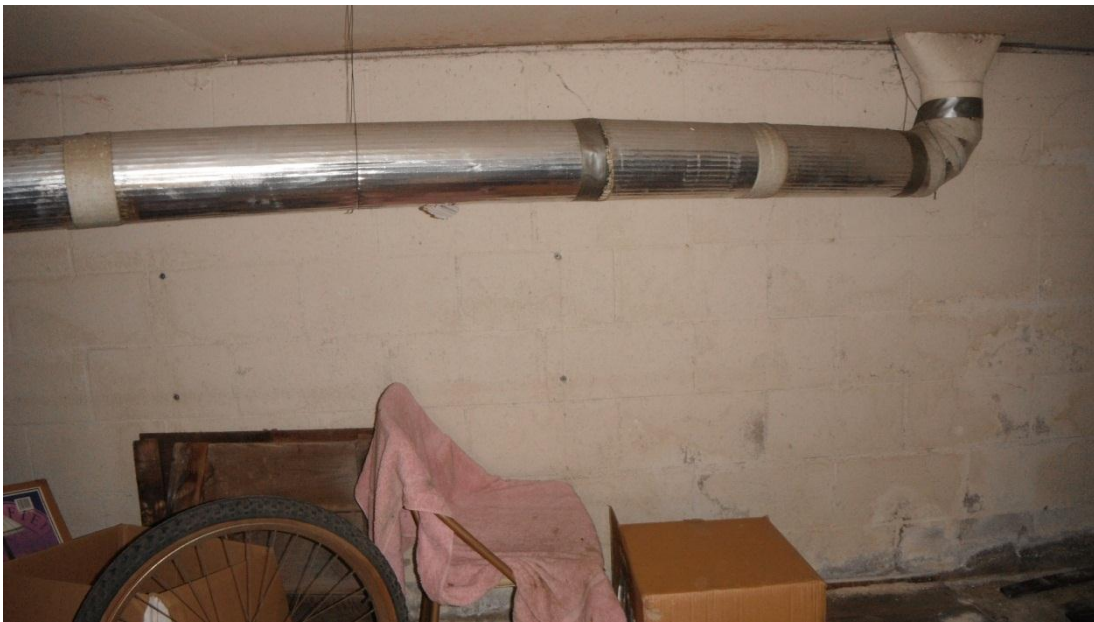
Asbestos insulation around heating pipes.
