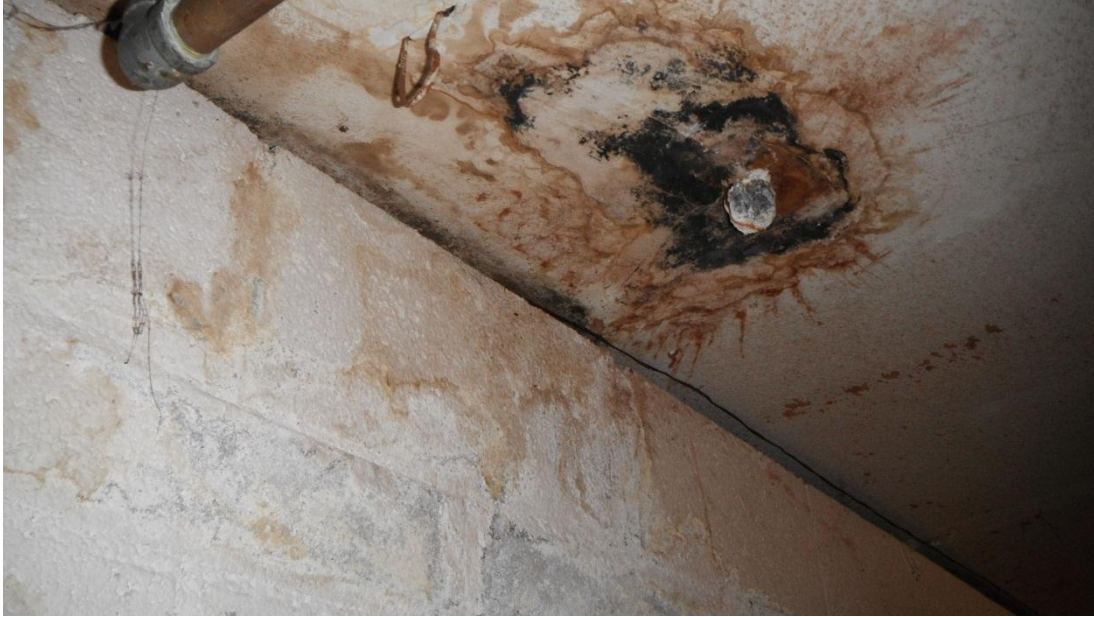
Galvanized water pipe leakage in the garage storage area.
