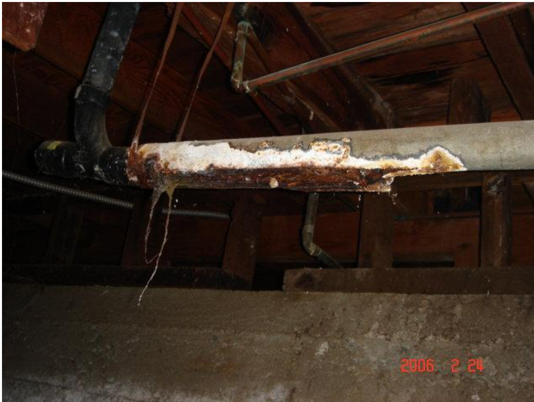
Corroded drain pipe, leaking to under the house.
