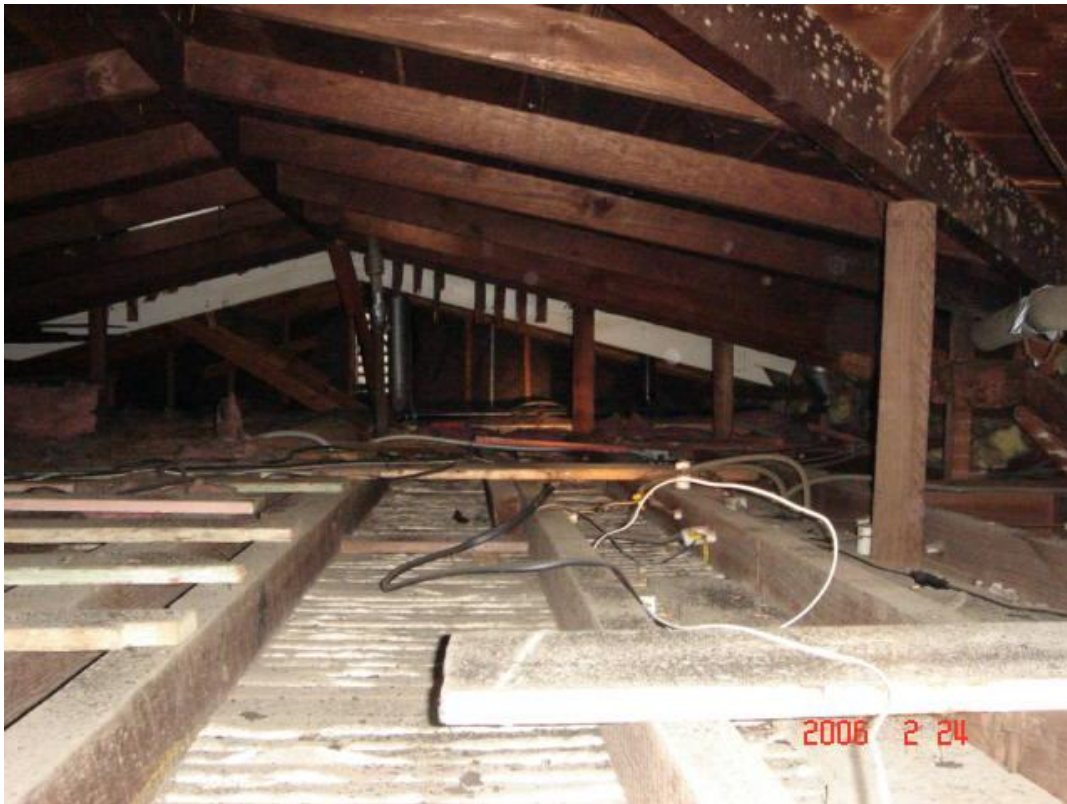
The attic, no insulation. Knob and tube wiring needing replacing.
