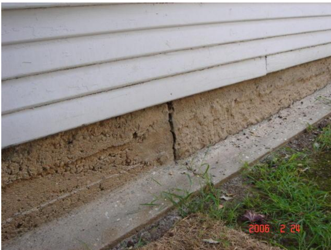
A crack in the concrete footing.
