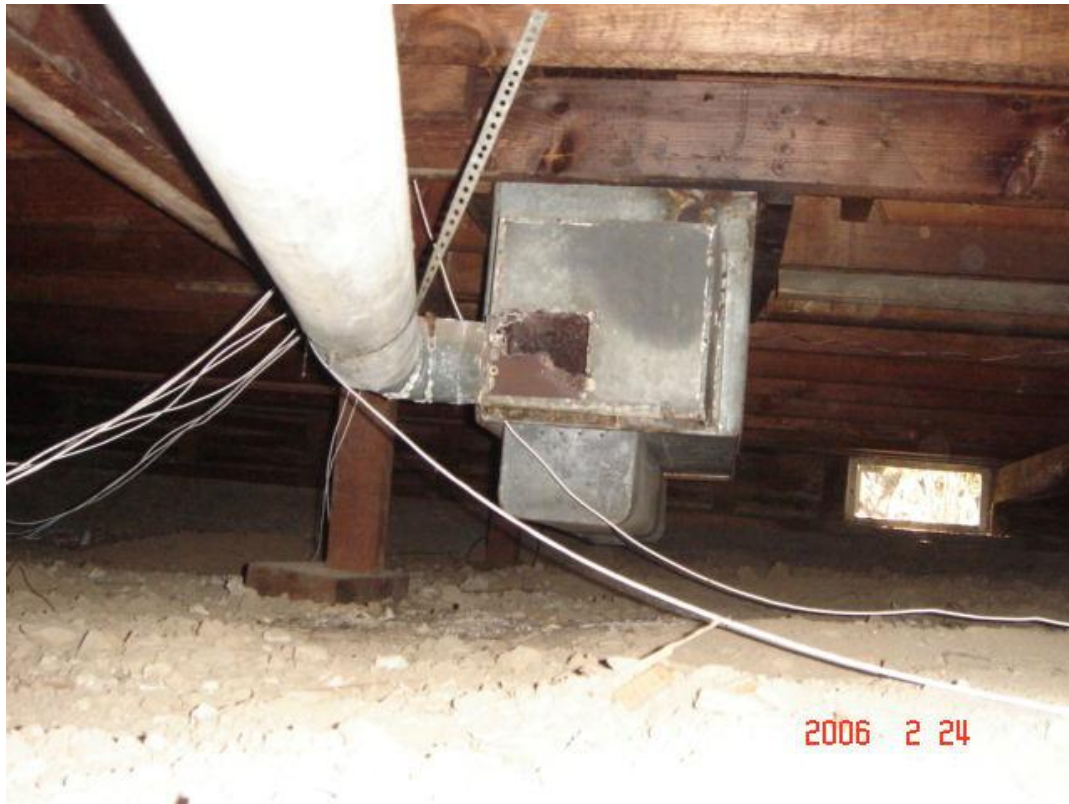
The rusted out vent box under the house.
