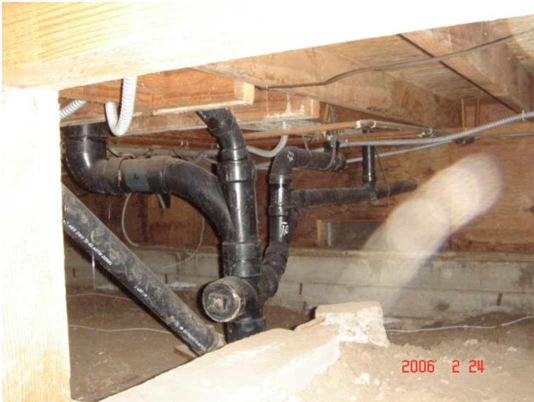
Improper drain fittings under the master bathroom.
