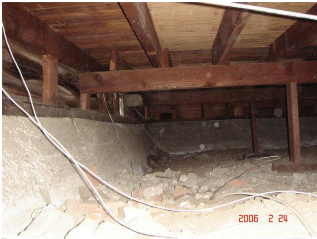
Lack of bolting, cripple walls and cracking to the foundation.
