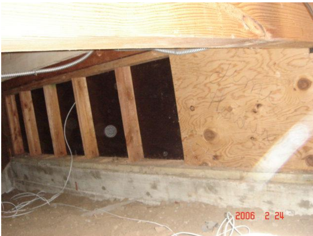
Partial incorrectly installed shear wall support.
