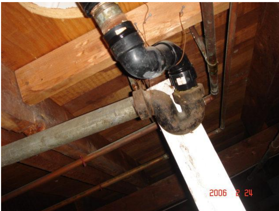
Improper drain fitting under the hall bathroom.
