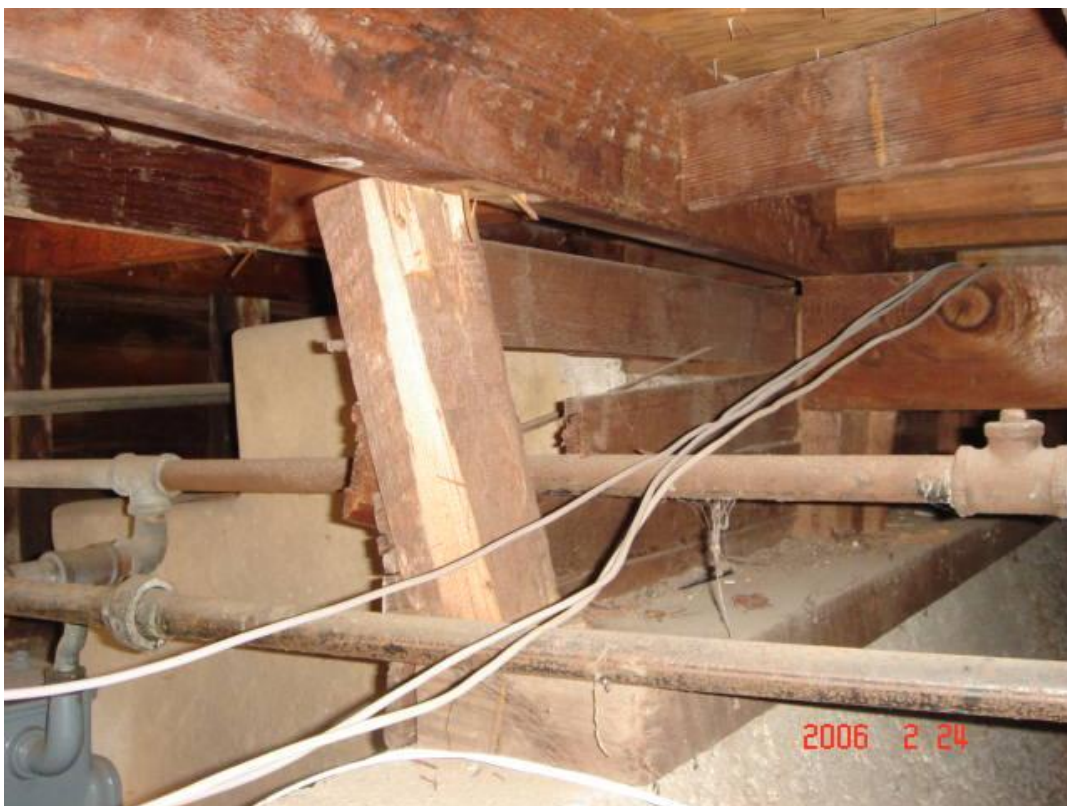
Loose cripple wall support.
