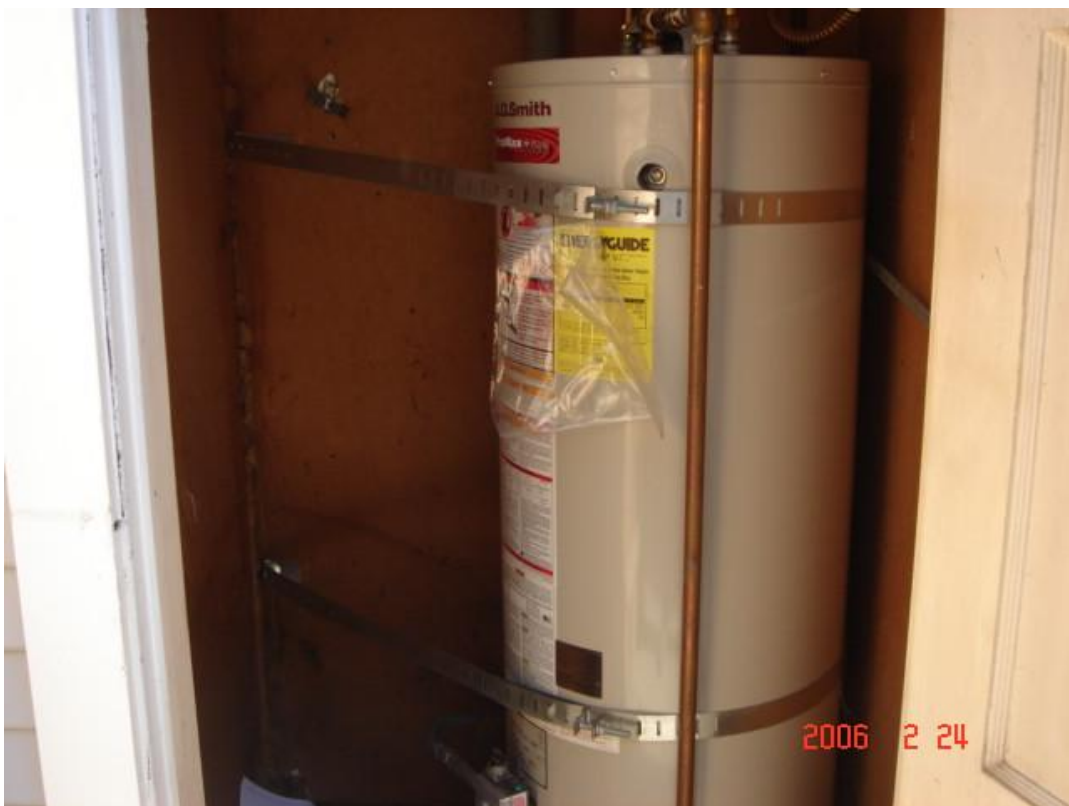
The earthquake strap to wide around the tank.
