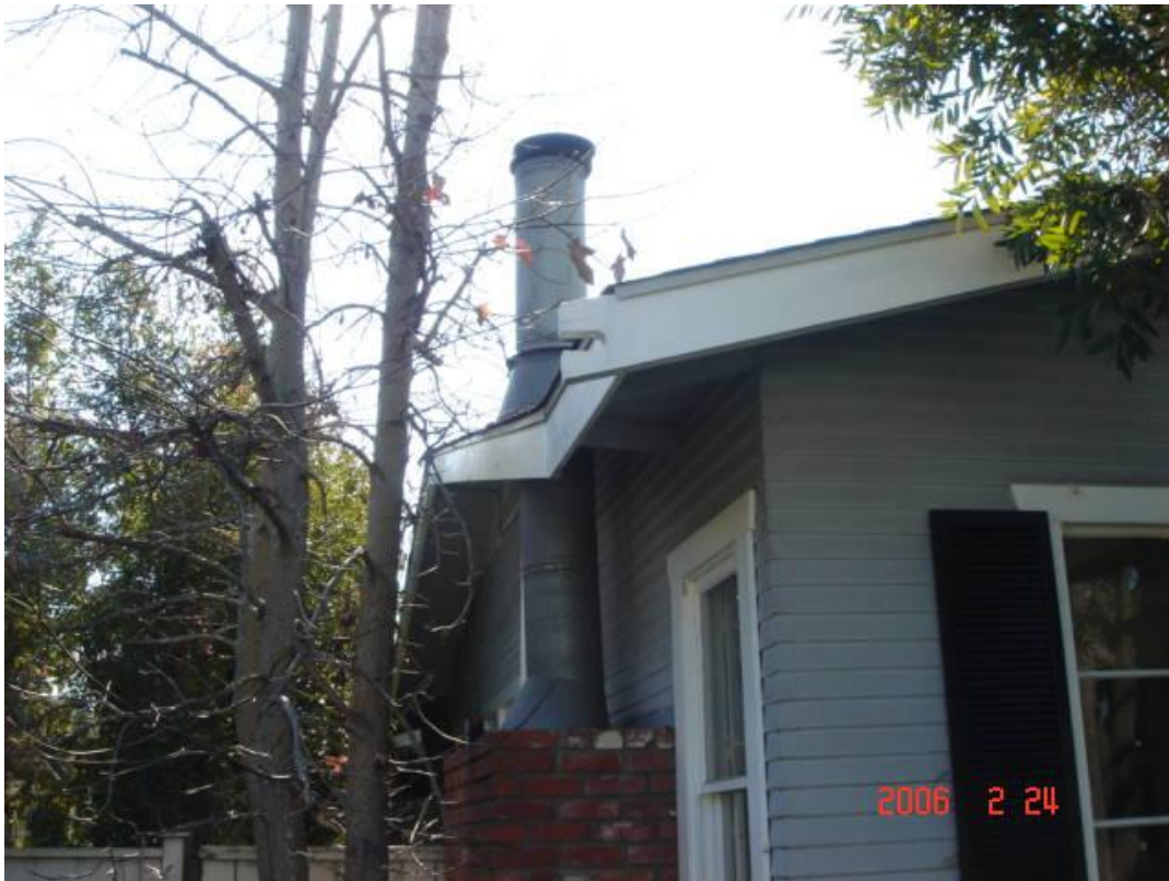
The fireplace and tree to close to the spark arrester.
