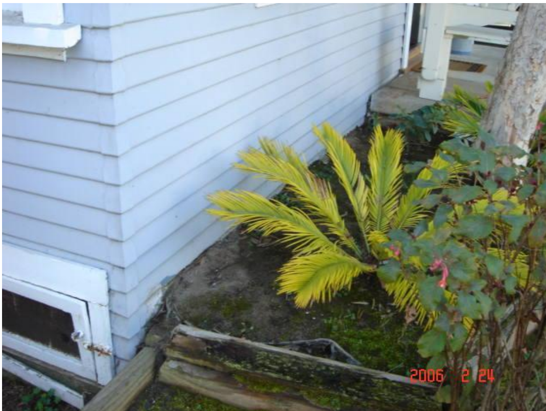
The planter box too close to the wood siding. (lead paint?)
