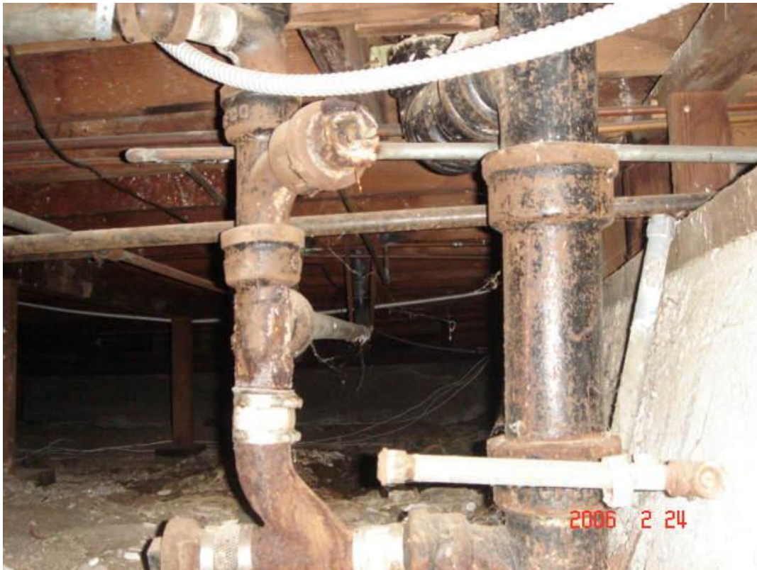
A section of corroded drain pipe.
