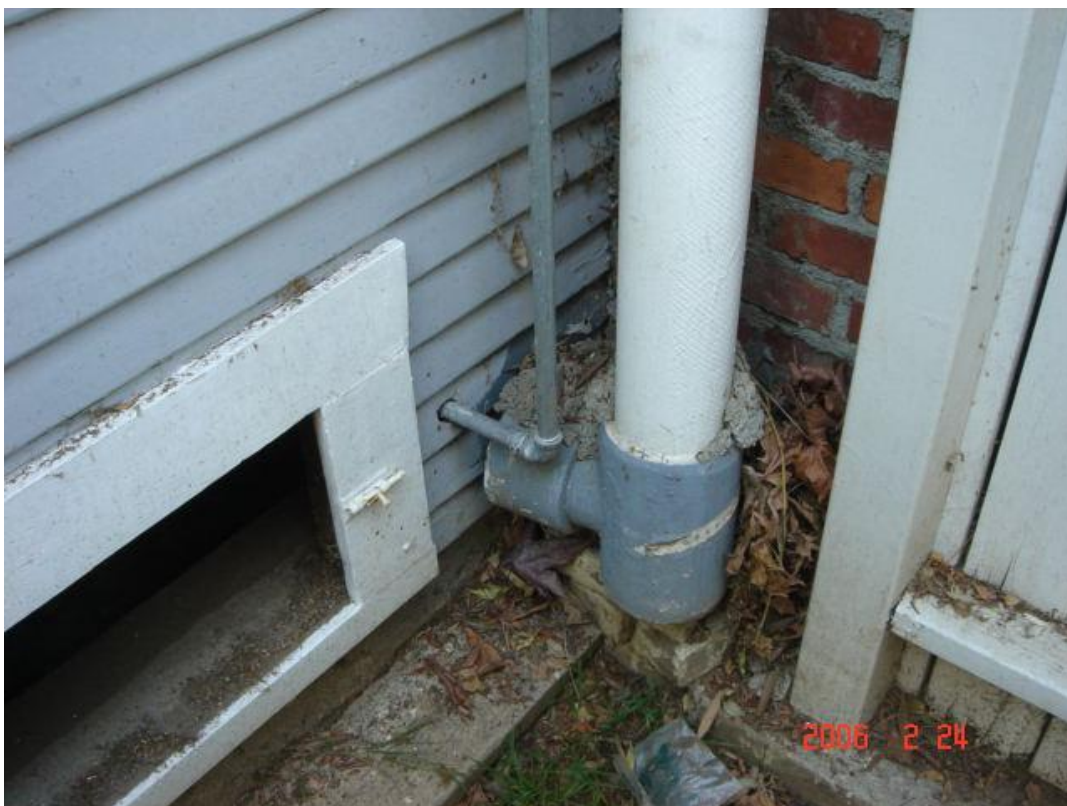
The disconnected floor furnace vent pipe by the fireplace.
