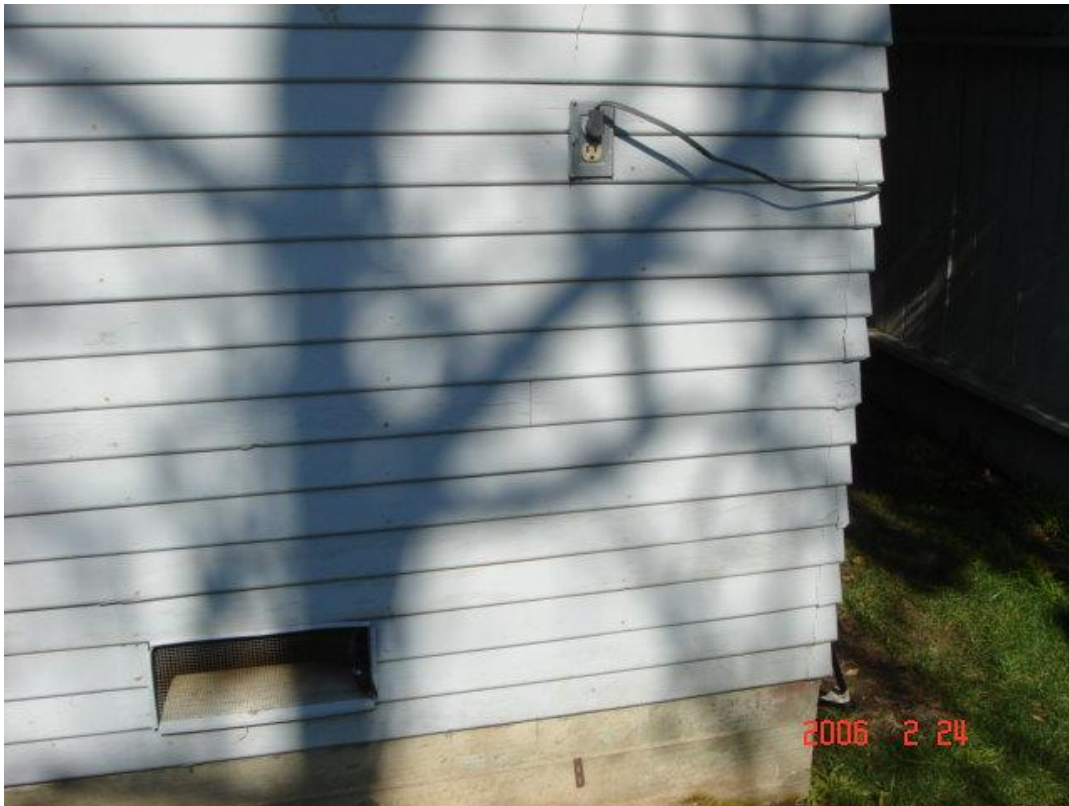
The unprotected outlet and wire at the foundation vent needing a box.
